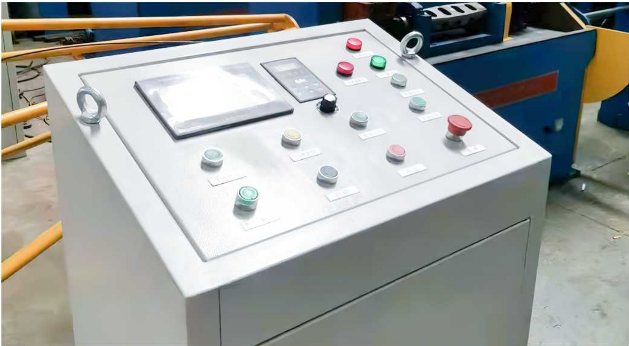
Electrical control cabinet
